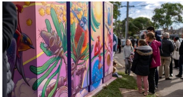
Neighbourhood battery installed in Fitzroy – June 2022. Photo credit ABC News
