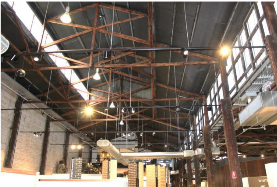
Figure 4 - Interior timber work showing roof trusses, posts and later brick party wall on east side
