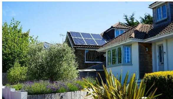
Solar panels on a home
