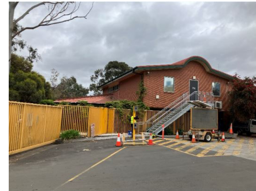
South Melbourne Operations Centre fire escape
