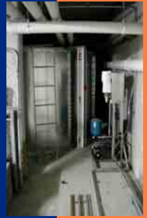
DETAIL OF WATER STORAGE TANK & PUMPS HOUSED IN THE BASEMENT CARPARK
