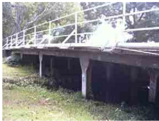
Reinforced concrete girder bridge at St Kilda Street, designed by John Monash
