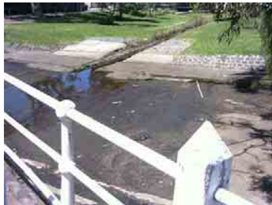
Looking south from Glenhuntly Rd bridge, showing start of the Elsternwick Main Drain
