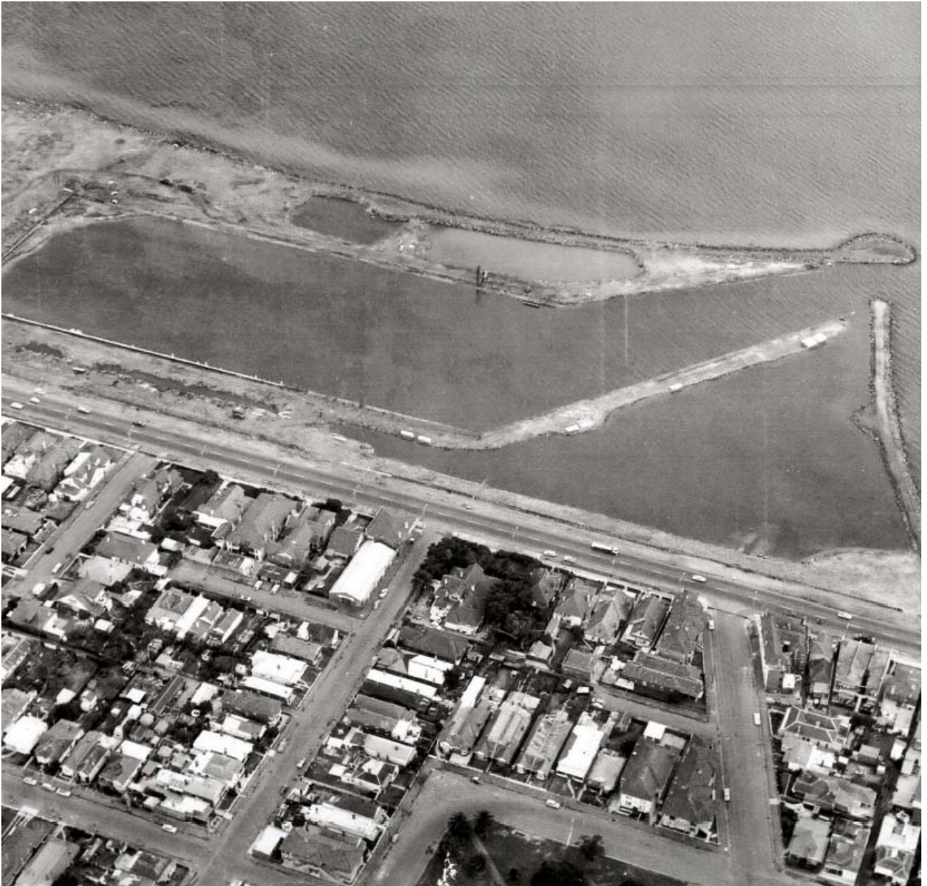
Plate 2 Beginnings of land reclamation for the St Kilda Marina (client provided, no date)
