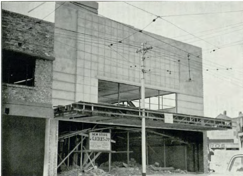
Figure 21 – Shows two buildings under construction in 1938, the Coles store at 156-160 Acland Street, as well as the building to left, part of the St Kilda Market site (now 181-89 Barkly Street). (Source: Colesanco 1938 , vol. 10, issue 47)
