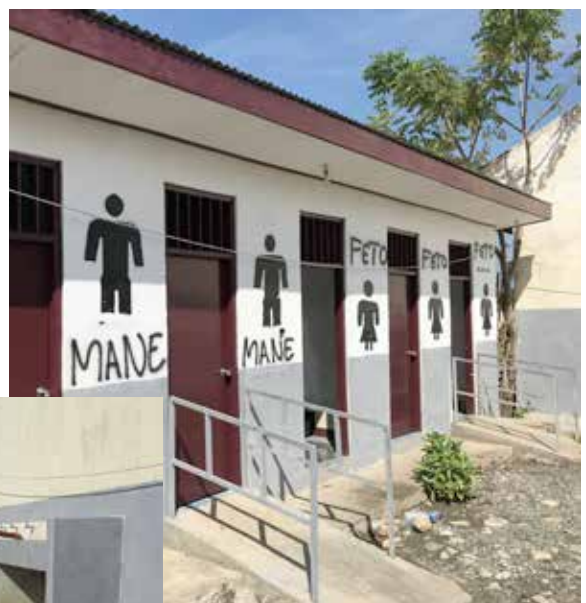
The toilets and wash basins at Suai Secondary School have recently been repaired, cleaned and painted.
