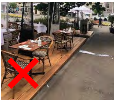
Figure 23: Platform is not flush with surround footpaths.
