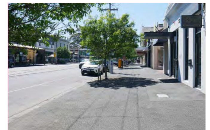
Image 29. Existing Park Street wide and extensive asphalt pavement
